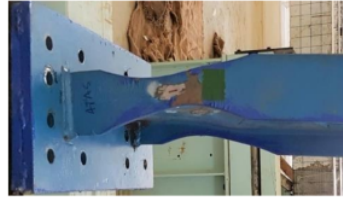
Fig. 9. Damage on RBSC-1 beam flange.
